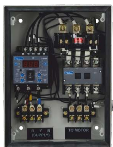
Interior View of MD Starter+ DOL Starter
