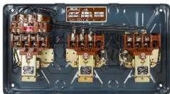
Interior View of MK2 SASD
