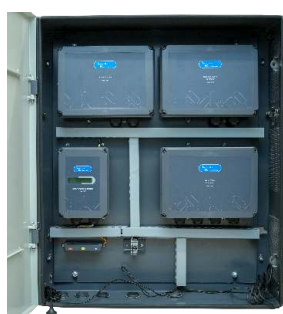
Interior View of xMasm10 - Wired Solution
